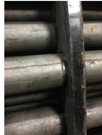
Support has cut into tubes. Flaw identified with IRIS.
