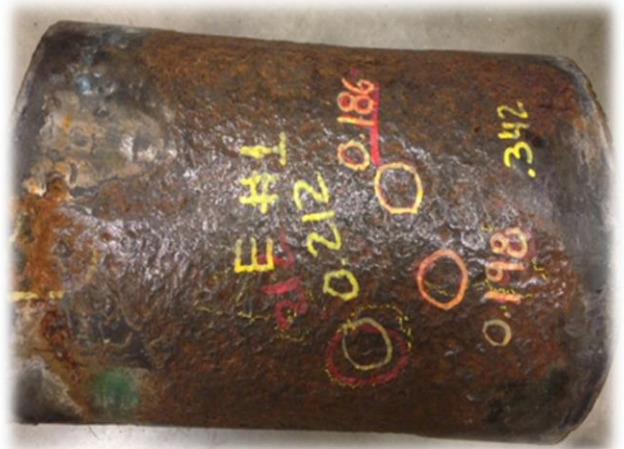
IRISNDT estimated 50% cross-sectional wall loss Follow-up results: 44% wall loss
