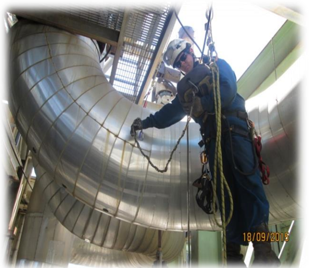
IRISNDT Technician Performing EMAT High Temperature Piping Thickness Measurements While Using Rope Access Technology (Dual Trained Personnel)
