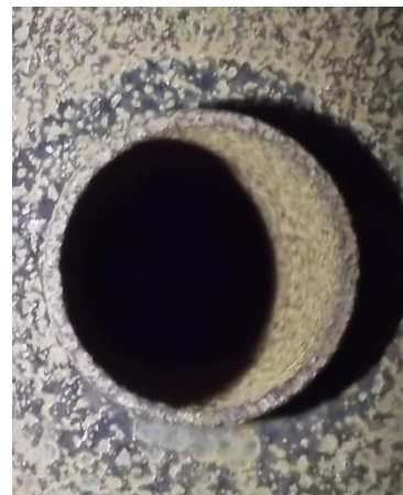
1.0 inch x 0.109 inch Fin Fan Tube Exhibiting Signs of General Corrosion
