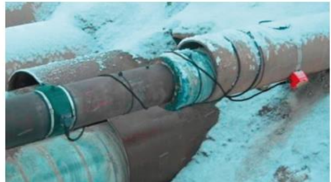
An overview of the 8" road crossing pipe monitored using gPIMS®.
