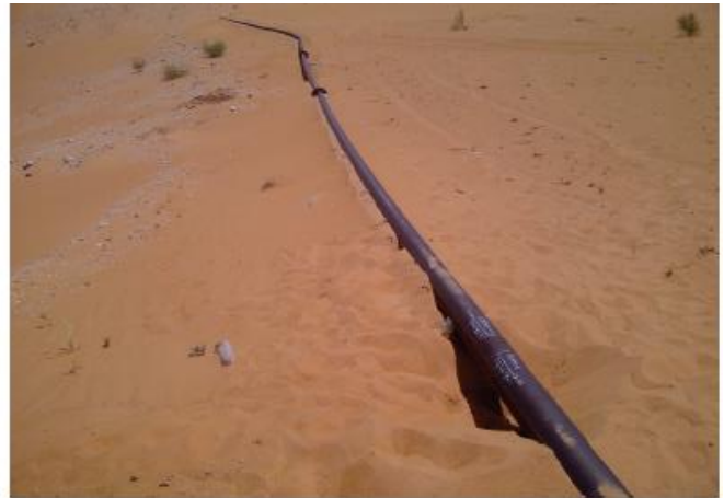
An overview of 6" flow line.
