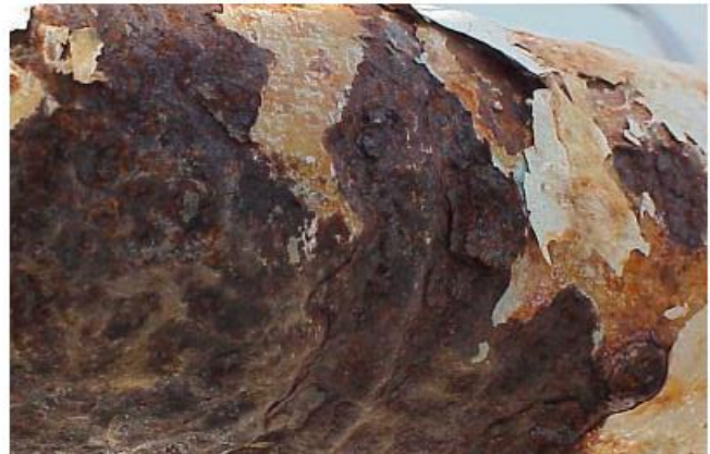
An area of severe corrosion on the 8" insulated pipe.
