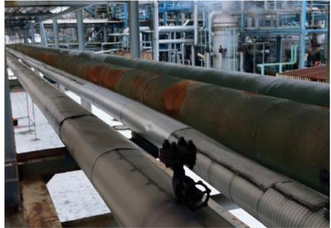
An overview of the 8" insulated pipe resting on the pipe rack.
