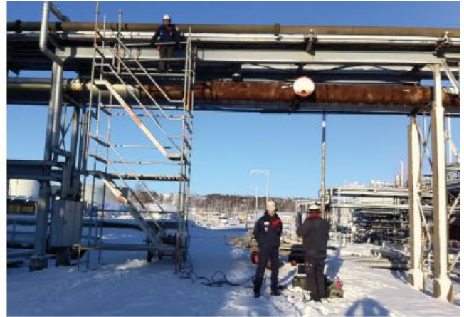
An overview of the piping at the jump-over location
