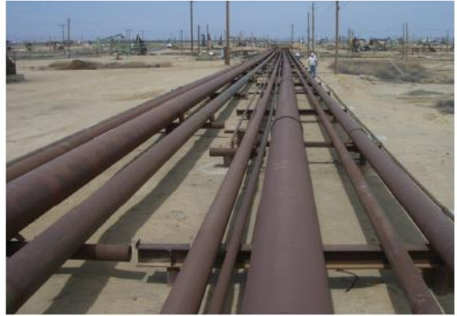
An overview of the 20" main gas gathering line.
