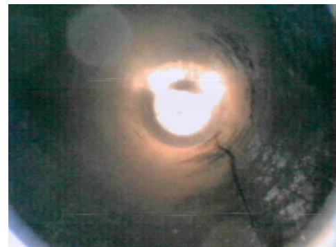
Through-wall crack in 1.0 inch x 0.109 inch stainless steel tube.
